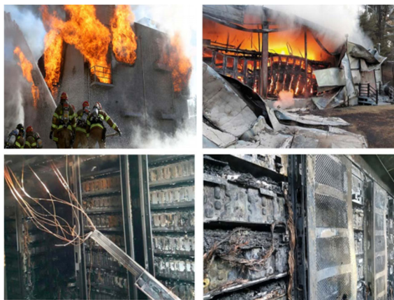
Figure 14: Fire Damage at Korean BESS Facilities 229
